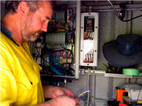
Brian Kirby (Bureau of Met) installing equipment for the Nauru Tide Gauge.
